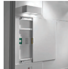
Sliding access doors
